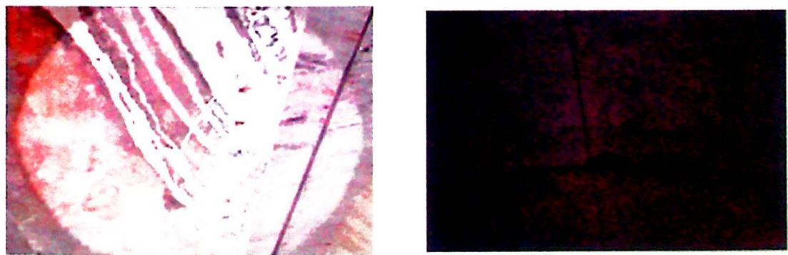
(a) 桥梁底破损
